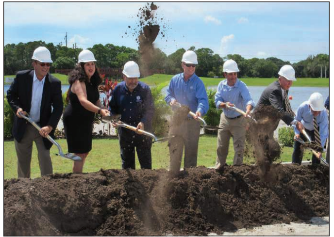
County administrator Tom Harmer, County Commissioners Christine Robinson, Al Maio, Charles Hines, Paul Caragiulo, Gulf Coast Community Foundation specialist Scott Anderson and Benderson Development president Randy Benderson participate in a groundbreaking ceremony for the finish tower at Nathan Benderson Park.
